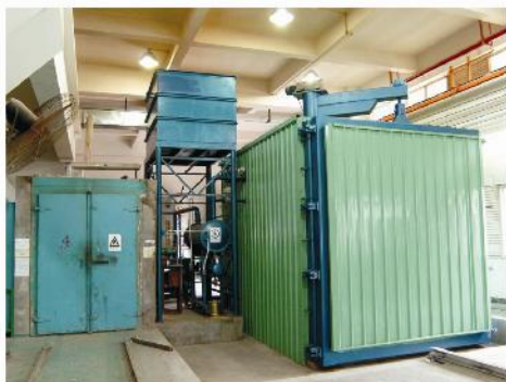
烘干炉 Drying Oven
